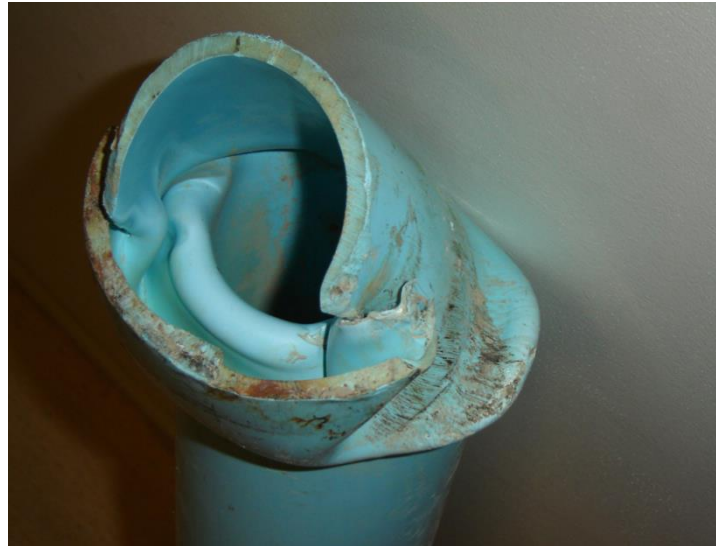
Figure IX - Ductile axial compression folding in PVC pipe, Gayhurst Road over bridge
