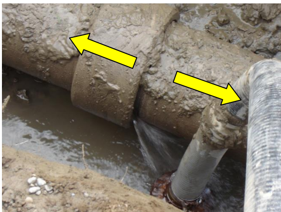
Figure III - Tension effects in AC pipe joint, Sewell Street Kaiapoi, axially aligned with the Darfield/Christchurch epicenter
