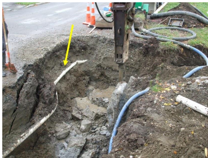
Figure VIII - Distorted but still operational, DN100 PVC-M water pipe with joint, Christchurch
