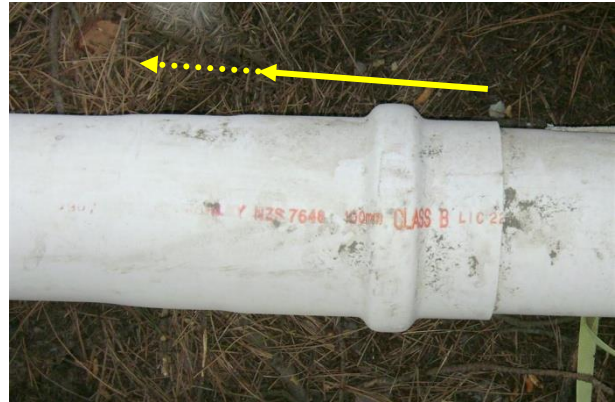
Figure VII – Compressed ductile joint movement in PVC-u water main, Christchurch
