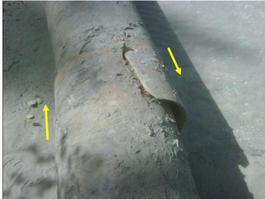
Figure VI - Compressed joint movement In CLS water main, Christchurch
