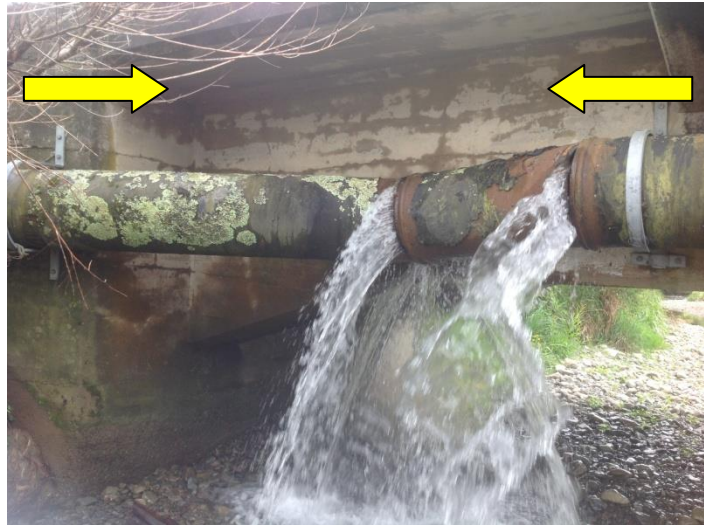
Figure V - Compression distortion and separation of gasketed joints in CLS watermain, axially aligned with the Eketahuna epicenter
