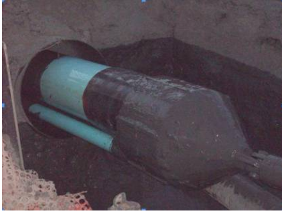
Figure 4. Pipe Bundle at Borehole Exit and Casing, also showing the arrangement with the manifold pulling shield and pipe pullhead configuration (Ostlund and Sarin (5)).
