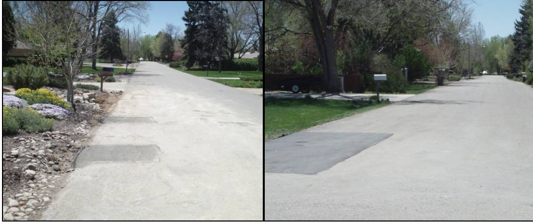
Figure 8. Final restoration in areas of pipe bursting. Asphalt patches shown in relation to rest of street.
