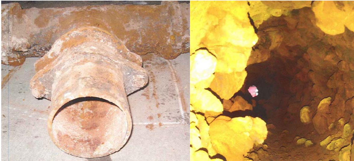
Figure 5. Typical water main in areas to be replaced, both outside and inside pipe showing tubercles (Botteicher et al. (6)).
